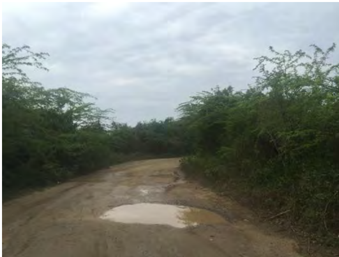
Photo 1. This is the beginning portion of the road. This area was not part of the erosion control project. Notice the water-created depressions.
