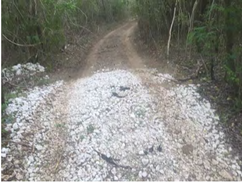
Photo 6. Check dam on connecting road to Panteón beach. This is the steepest road and of highest elevation. It was identified as the main producer of sediments and runoff speed during substantial precipitation events.
